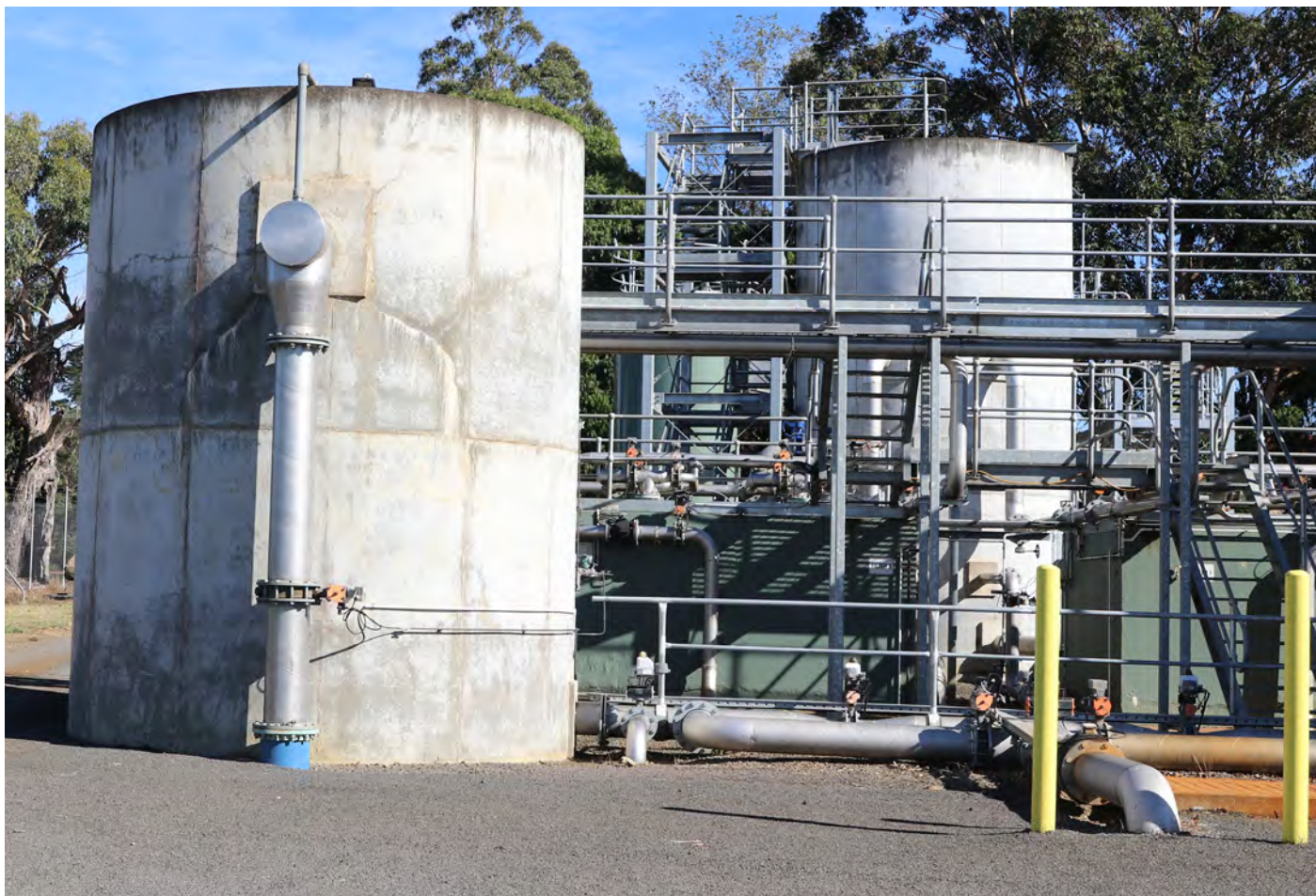
Casterton Water Treatment Plant
