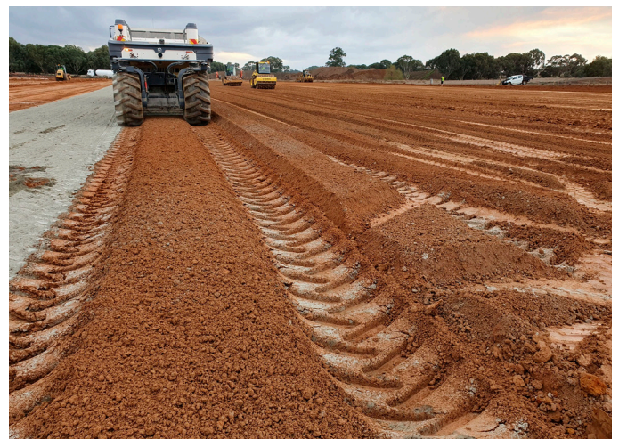
Biosolids drying area, Hamilton.
